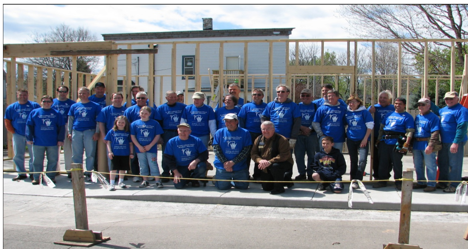
Family and friends of St. John's Lutheran Church in Brookfield gathered April 18 to raise the first walls of the new storage facility.
